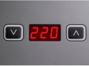
Centralized temperature control
